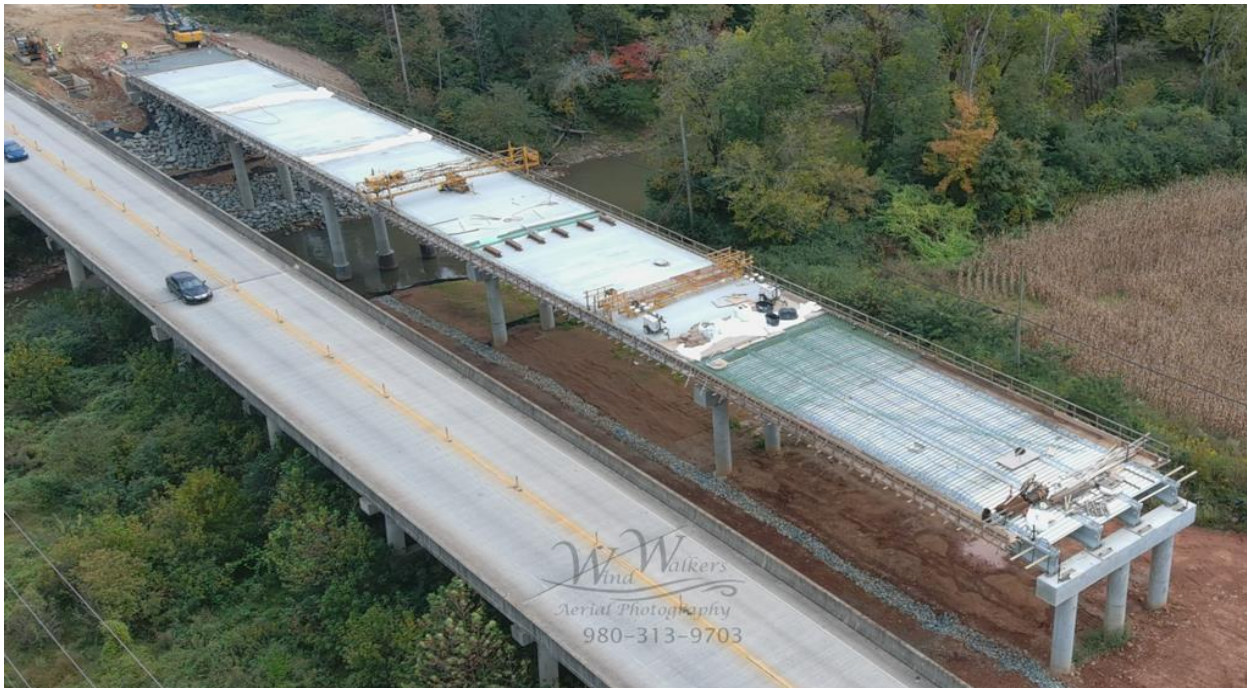
Figure 11. NC 24/27 and Rocky River bridge construction project. Photo courtesy of Wind Walkers Aerial Photography.
