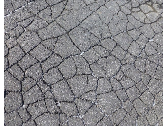
Figure 6 – Example of Crack in Asphalt Pavement
